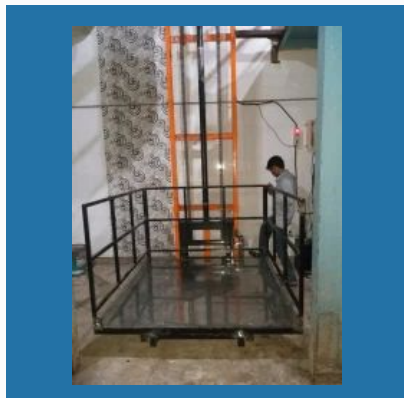
Hydraulic Goods Elevator
