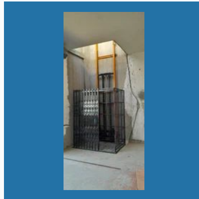
Hydraulic Lift Material Goods
